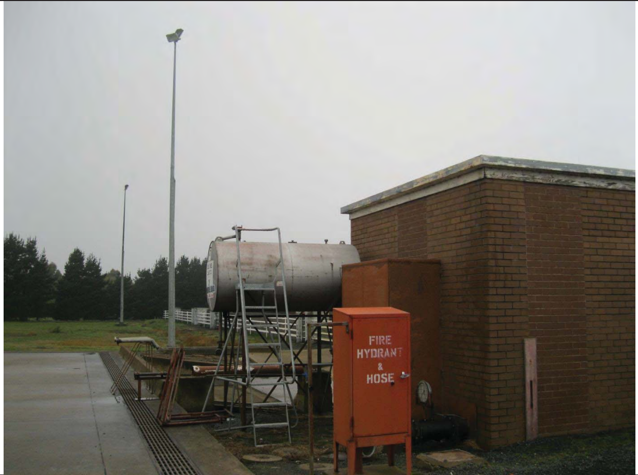
PLATE 3 Aboveground Storage Tank Area 2 (Feature 23b) looking east
