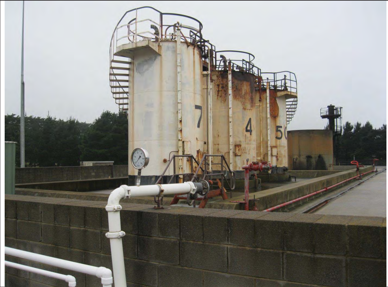
PLATE 6 Above ground Water Storage Tanks 1 (Feature 57a) looking north-east
