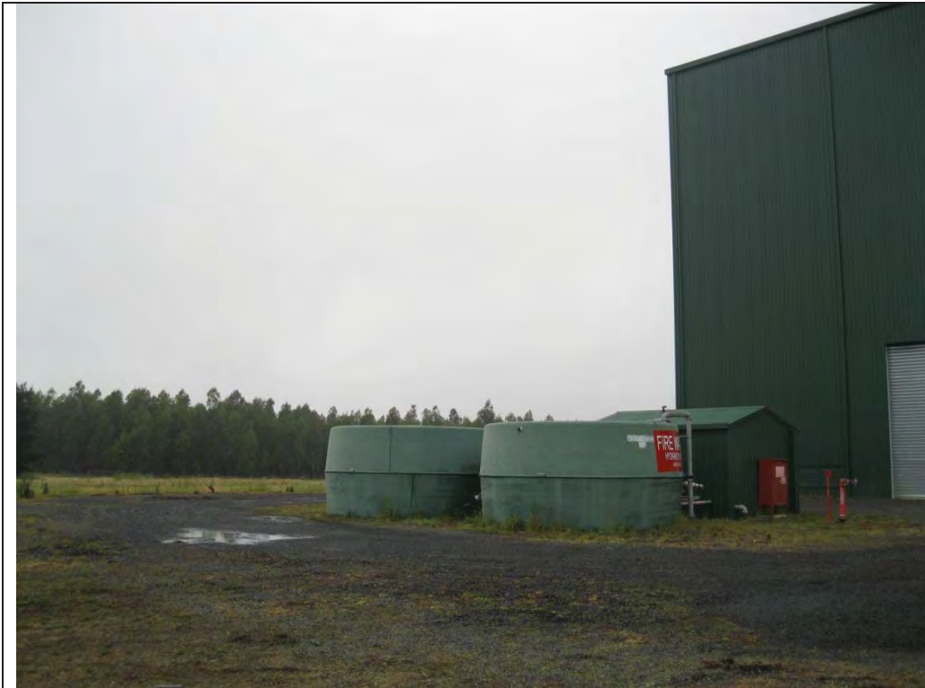
PLATE 5 Rain Water Tanks
