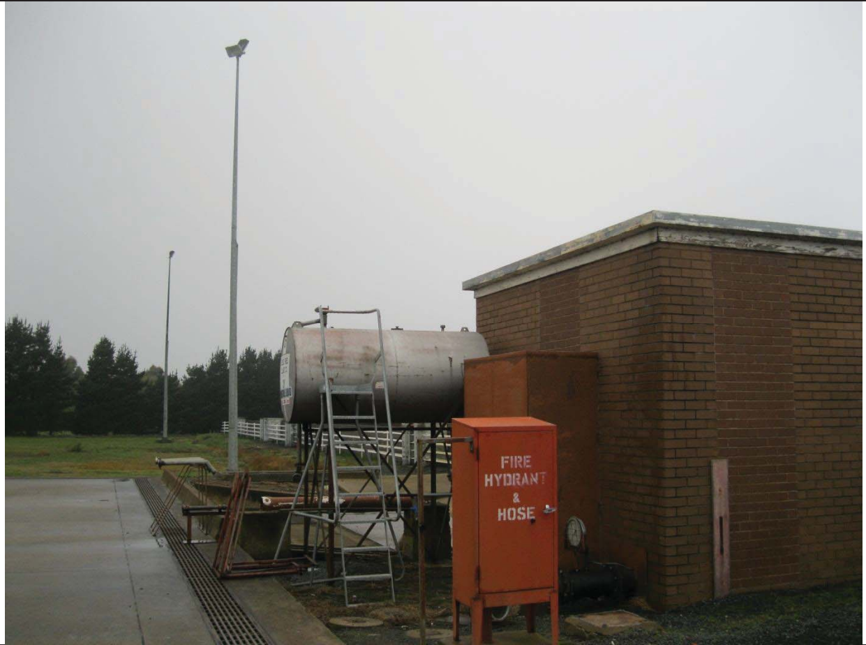
PLATE 4 Aboveground Storage Tank Area 2 (Feature 23b) looking east
