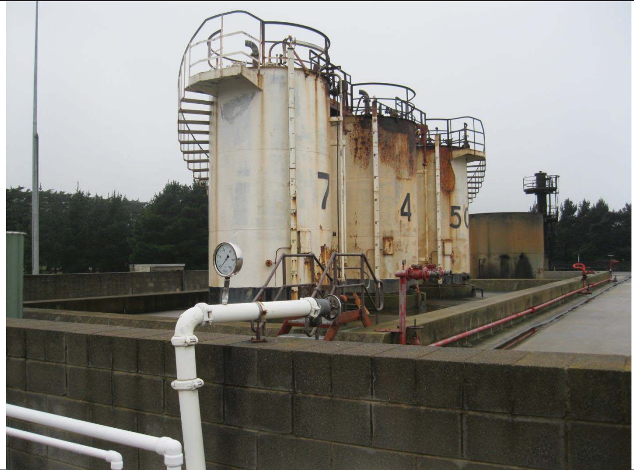
PLATE 7 Above ground Water Storage Tanks 1 (Feature 57a) looking north-east
