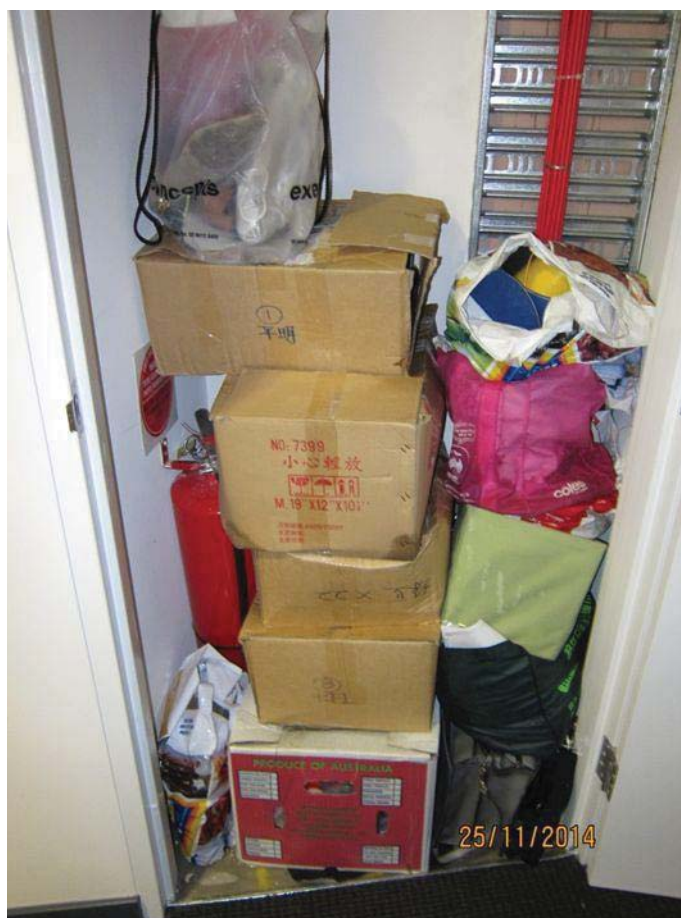
Figure 13 - Fire extinguisher cupboard on Level 6.
