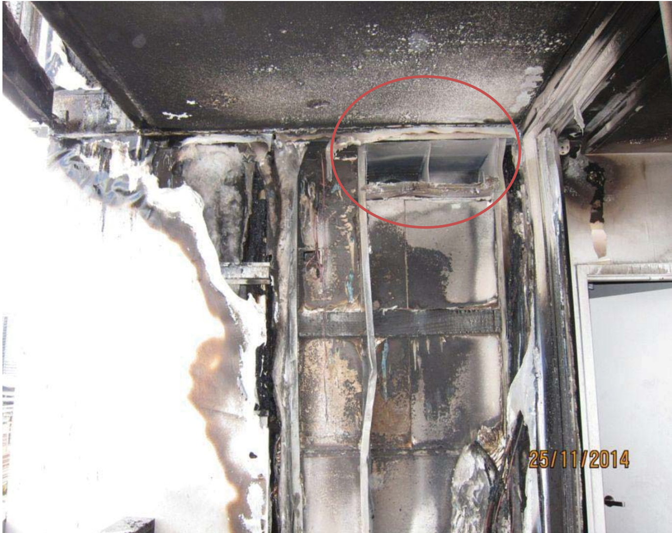
Figure 19 - Apartment Exhaust Duct
