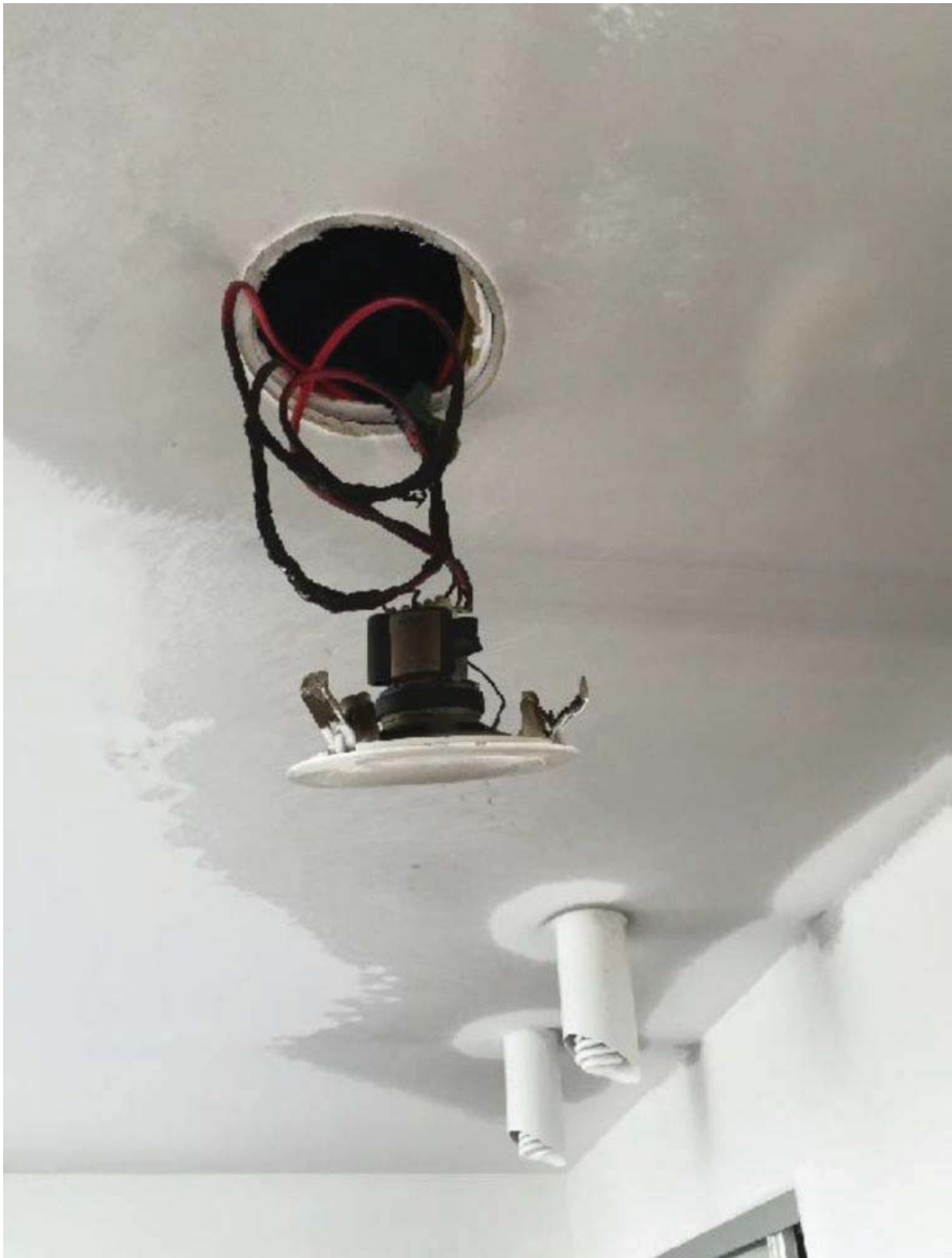
Figure 20 - EWIS Speaker and wiring
