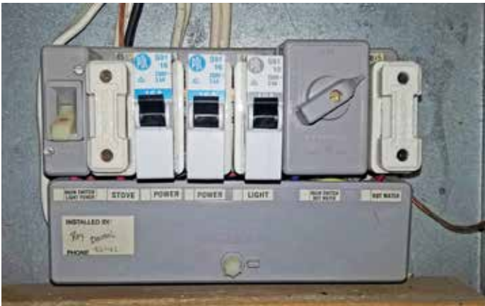
↑ A typical 1970s switchboard. This type of switchboard was commonly used from the late 60s to the late 80s. It is generally cheaper (and better) to change it to a modern board with combination safety-switch/circuit breakers than attempt to modify it! Also, if upgrading the supply to the house, it must be replaced.
