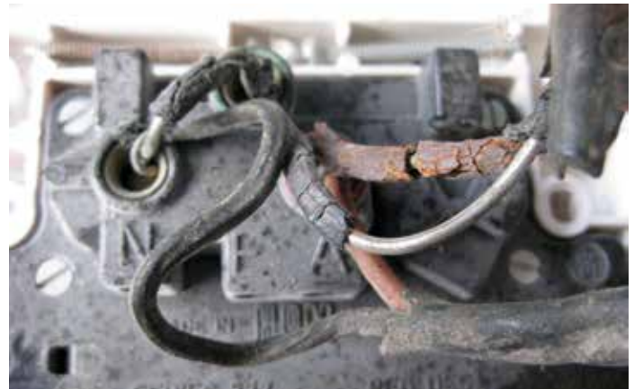
↑ Decomposing VRS (Vulcanised Rubber Sheath) cable at a power point. This must be replaced when any electrical work, such as fitting an EVSE, is done.
