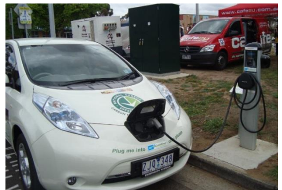
Figure 8: Moreland EV charging (source: Sustainable Fawkner)
