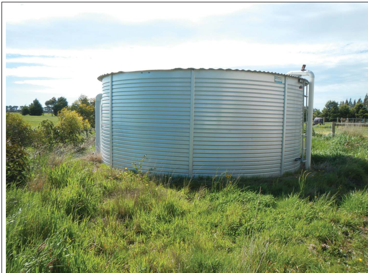
PLATE 12 Rain Water Storage Tanks (North tank). (Source of WT04)
