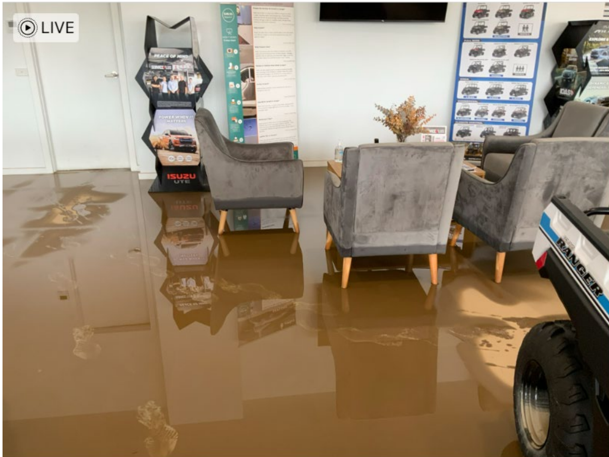
The photo above shows depth of flooding as indicated on watermark on chairs and impact on new car showrooms. Photo taken after peak flow has subsided
