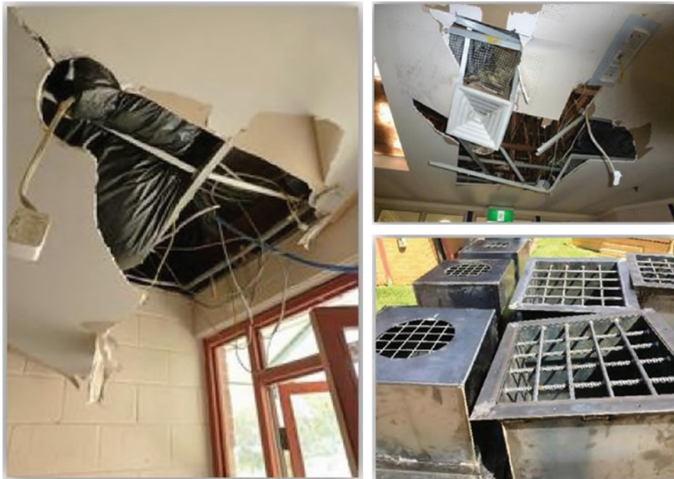
Figure 8.1 Ceiling damage and new steel vent covers at Parkville Youth Justice Precinct.
