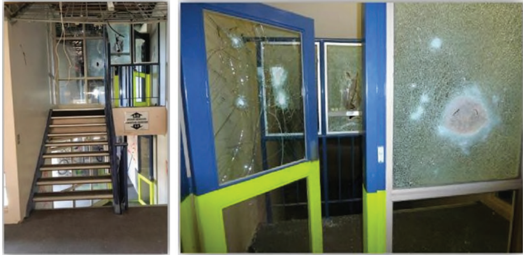
Figure 8.2 Damage to a residential unit at Parkville Youth Justice Precinct
