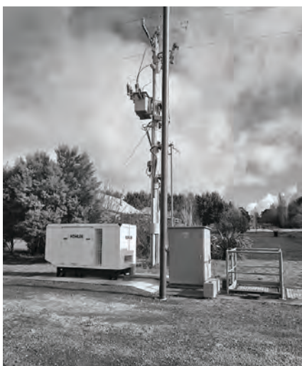
Figure 3. New back-up generator for a sewer pump station in Tylden
