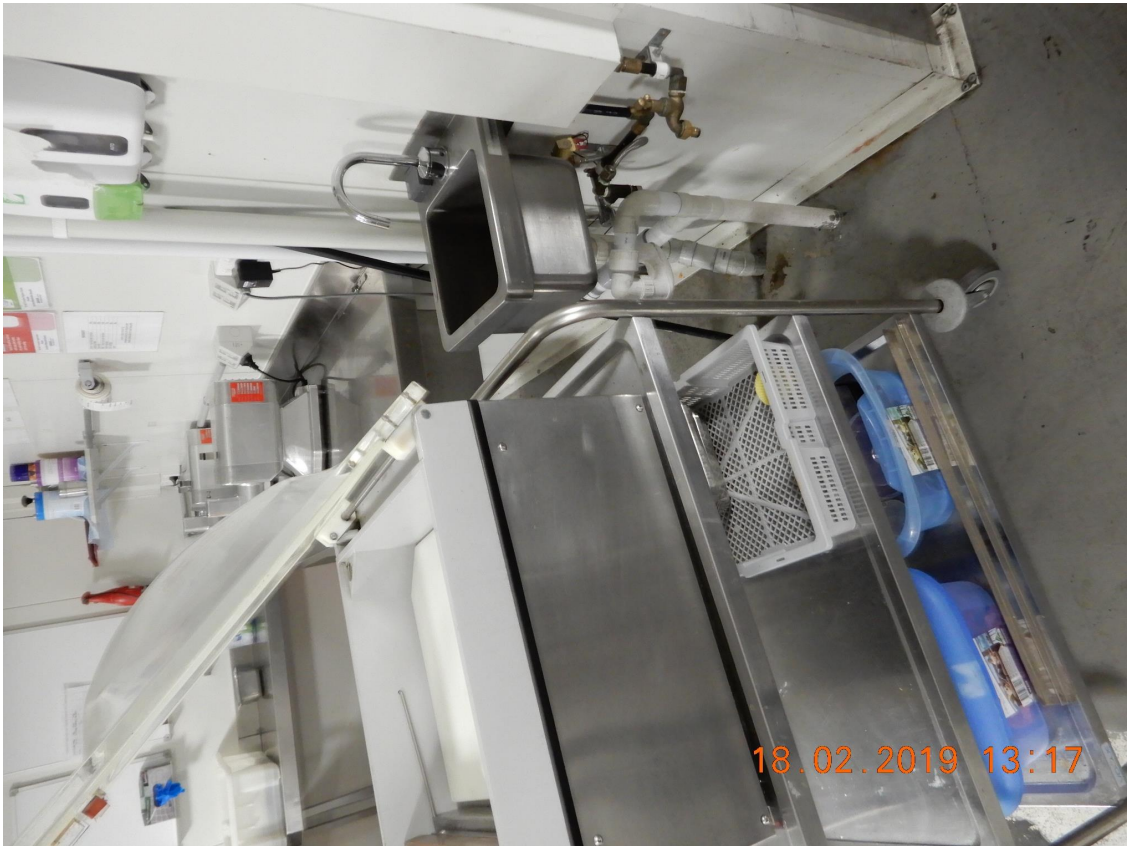
EG84: Photograph of hand wash basin with vacuum sealing machine in front of it at mincing station in Plating/Packing Area. Photograph: Officer E. Garlick. Date: 18 February 2019
