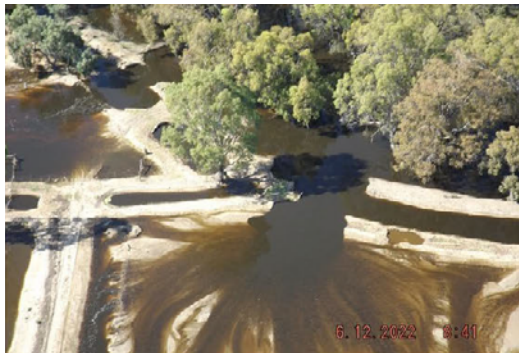
Levee breach in Gannawarra Shire
