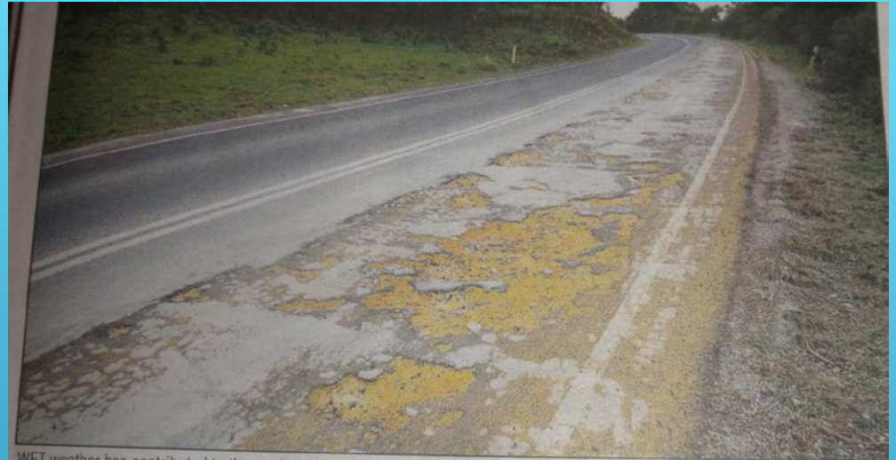
WET weather has contributed to the road surface breaking up.
