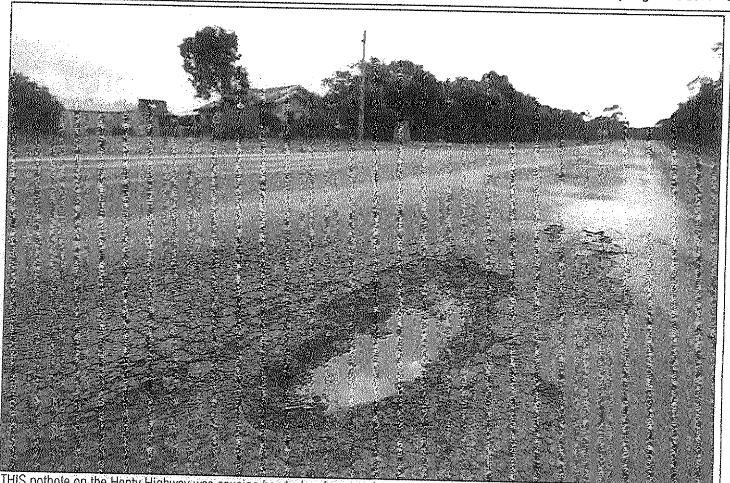
THIS pothole on the Henty Highway was causing headaches for motorists on Monday.
