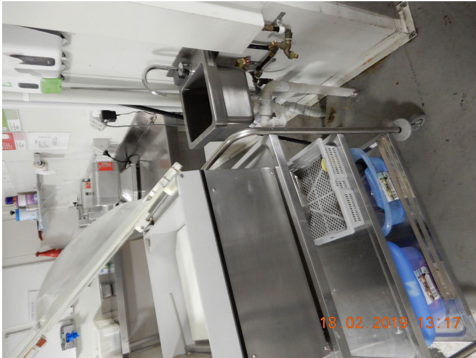
EG84: Photograph of hand wash basin with vacuum sealing machine in front of it at mincing station in Plating/Packing Area.
