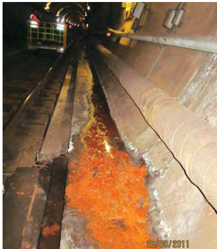
Figure 1: Burnley Loop – severe leached rust water on walkway
