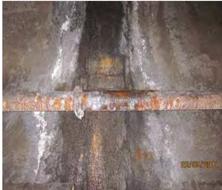
Figure 4: Burnley Loop - severe corrosion on fire line
