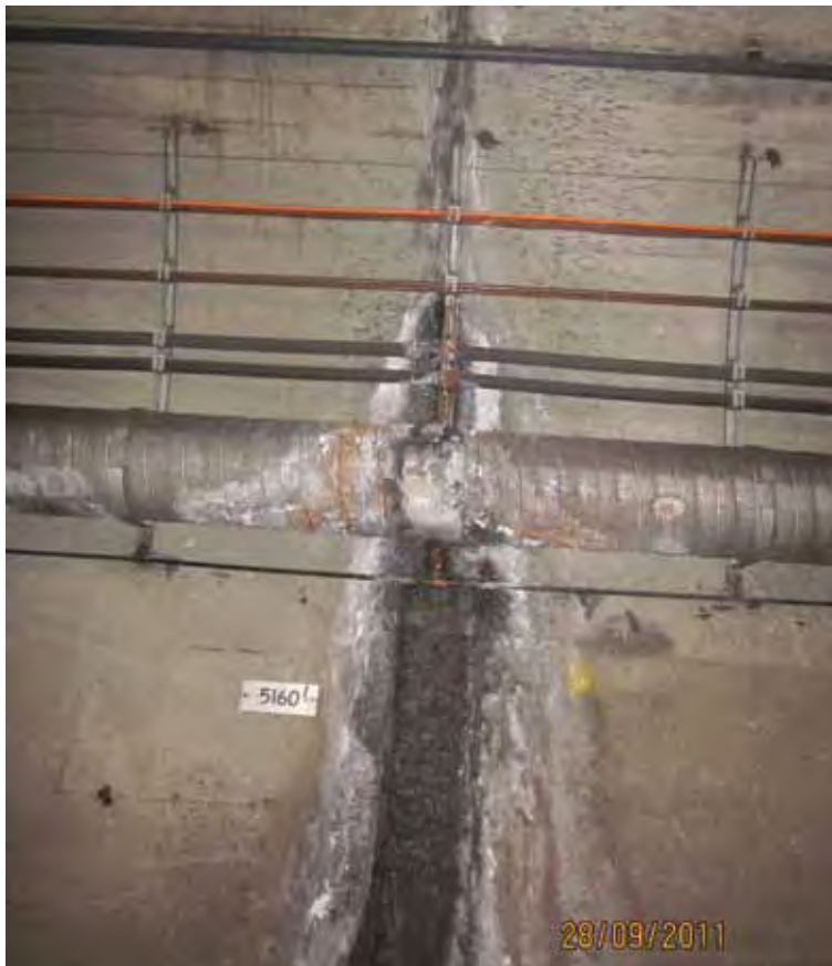
Figure 2: Burnley Loop - high wall cracking and leaching of concrete
