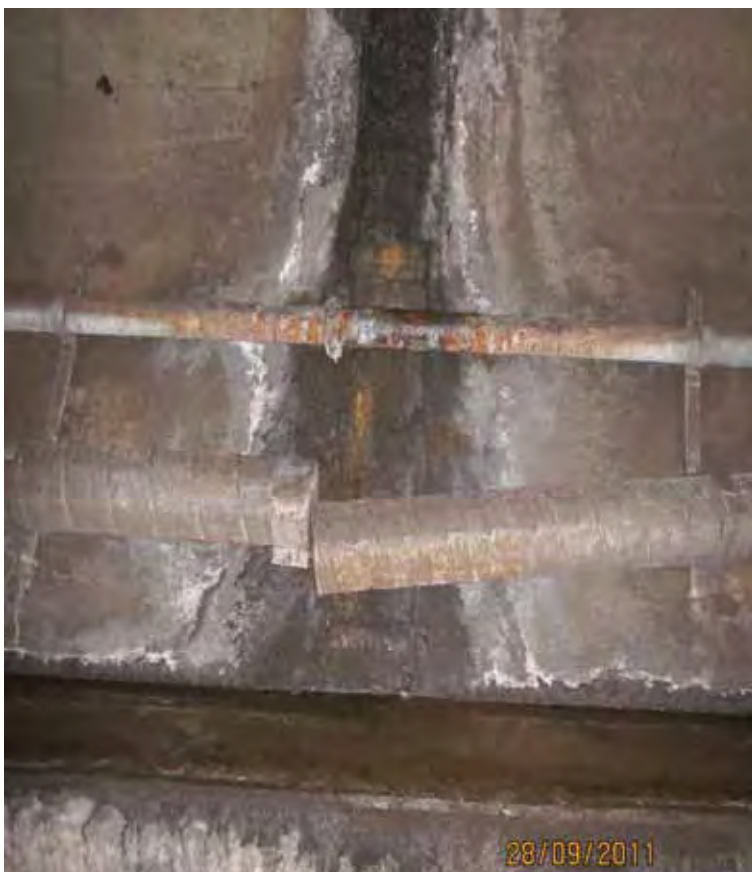
Figure 3: Burnley Loop - corrosion
