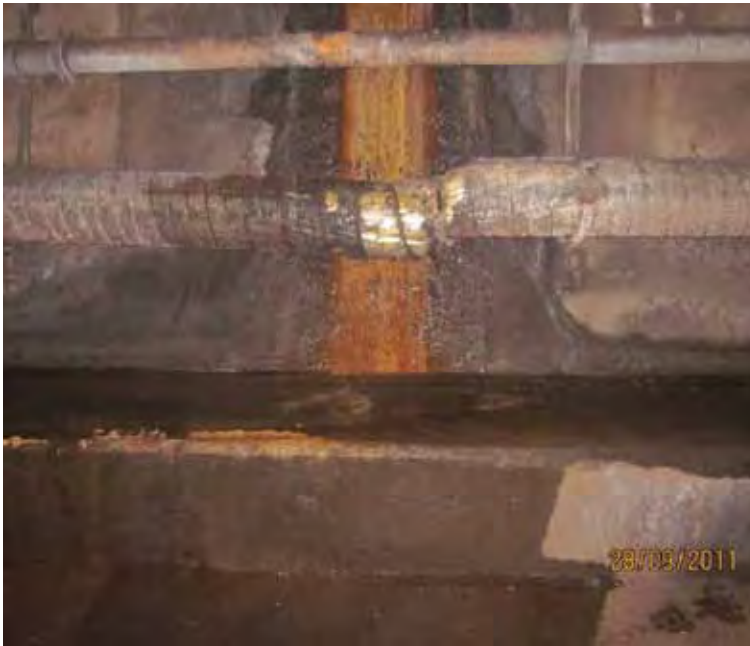
Figure 6: Northern Loop - severe corrosion and leaching
